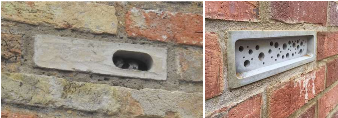
Figure 67 – Examples of artificial nests: swift bricks and bee bricks can be of particular benefit in an urban context
