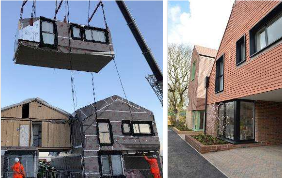
Figure 92 - Beechwood West, Basildon: A new neighbourhood of over 250 volumetric family houses utilising factory-built modular technology offering a choice of housing typologies, layouts and external finishes, precision engineered in an efficient and sustainable way with a significant reduction in construction waste compared with traditional build methods.
